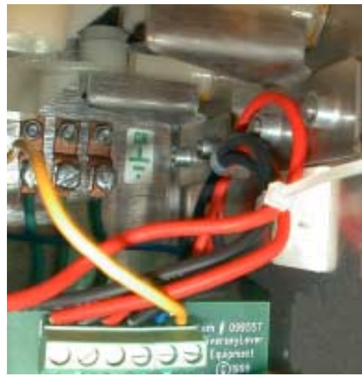
Figure 2. Pump terminal wires secured with wire harness and tie wrap.
