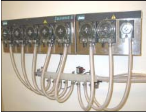
8-Port Summit E manifold, mounted beneath dispenser
